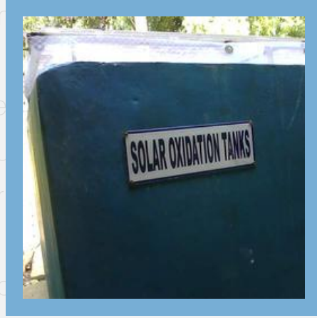
Solar Oxidation Arsenic Removal System
